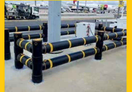
Atlas Double Traffic with reflective striping protecting an airport mast and electrical unit.
