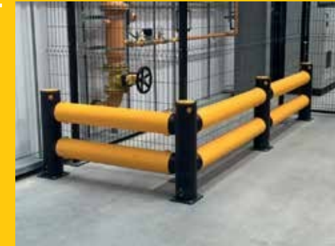
iFlex Double Traffic protecting main sprinkler system in a food processing factory.
