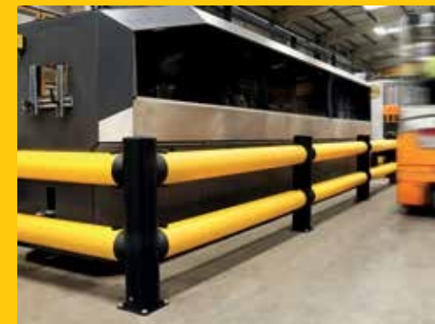
eFlex Double Traffic shielding equipment in a manufacturing facility.
