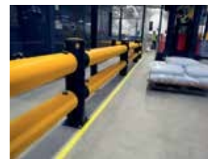
14 Double Traffic Guardrails
