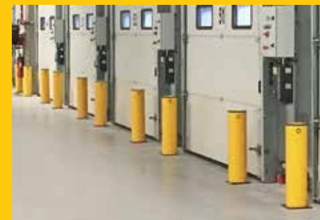
Bollards shielding door frames and shutter runners in a newly built warehousing and distribution center.
